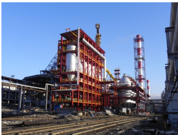
Figure 1. Dry gas cleaning.
